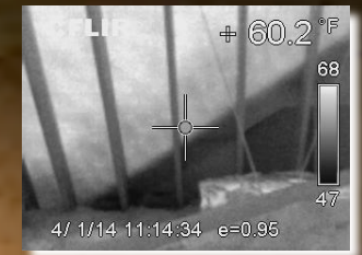
IR image of same location shows dramatic temperature variation: a contributing factor for cause of mold.
