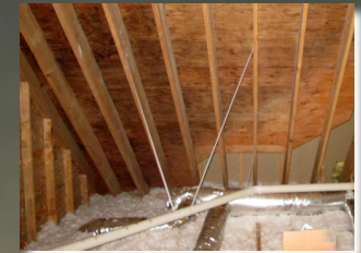
Attic shows well-defined demarcation of mold vs. clean.
