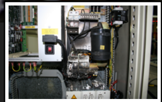
Electrical panel fires can result from multiple causes.
