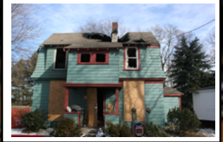
Woodburning appliance fires can cause disastrous damage.
