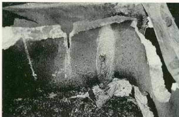
Chamber damaged by cleaning tools
