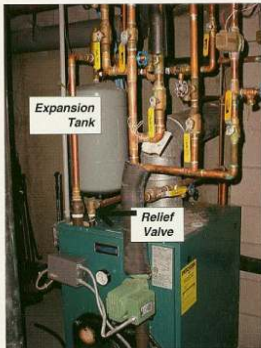
Hot water heating system
