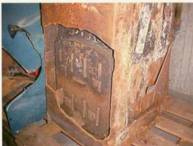
Burst expansion tank
