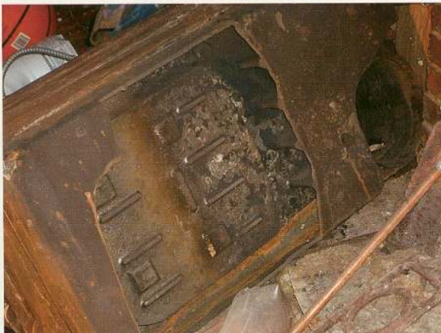
(Above) boiler section damaged due to BLEVE
